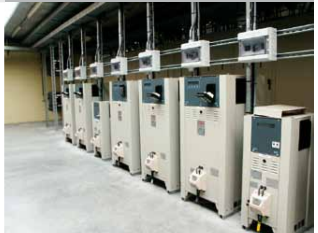
Fig. 2: MCR 3 in substation
